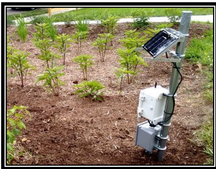
Fig. 5.21 Moisture Monitoring System
